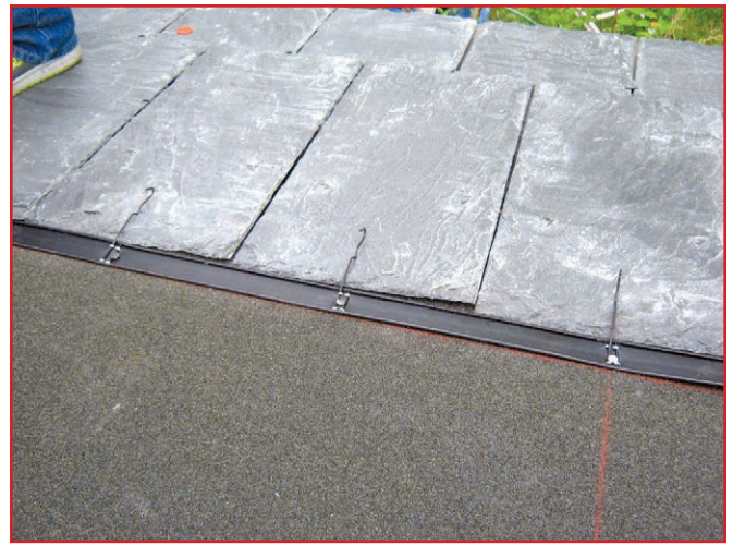
Figure 6 – Qwik Slate installation in progress. Photo courtesy of Brian Chalsma, The Roofing Company, Hampton, VA.
